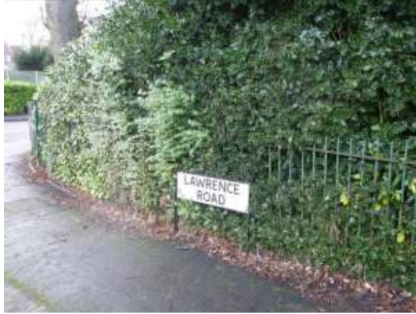
Historic railings in need of maintenance
