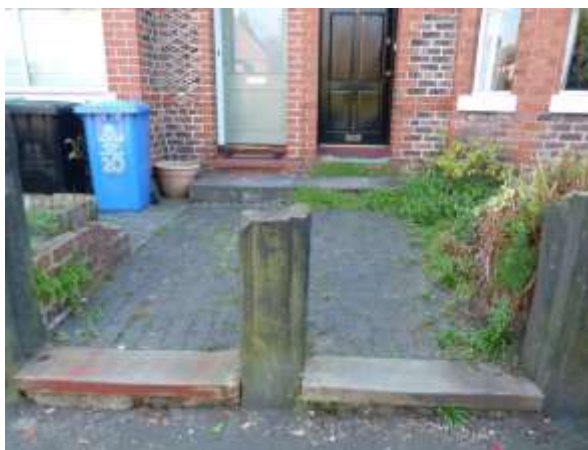
Damaged original stone gateposts and original brick pathways on Weldon Road
