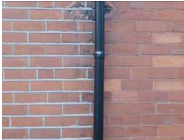
Inappropriate ribbon pointing to No. 3, with correctly recessed pointing to No. 5
