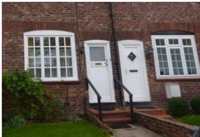
An original style window and door on the left; on the right, a modern replacement door in a similar style and thick-framed UPVC windows.
